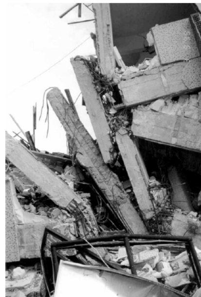
Beam-column joint shear failure
