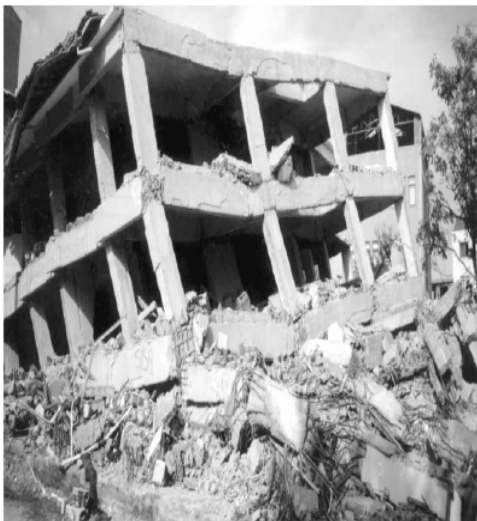
Beam-column joint shear failure
