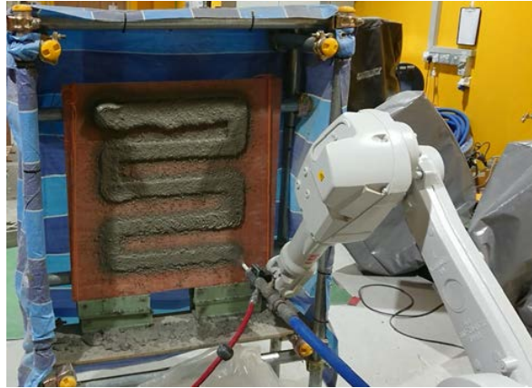
Figure 3 Experiment setup consist of robotic arm, cementitioul pump with hose and high pressure air
