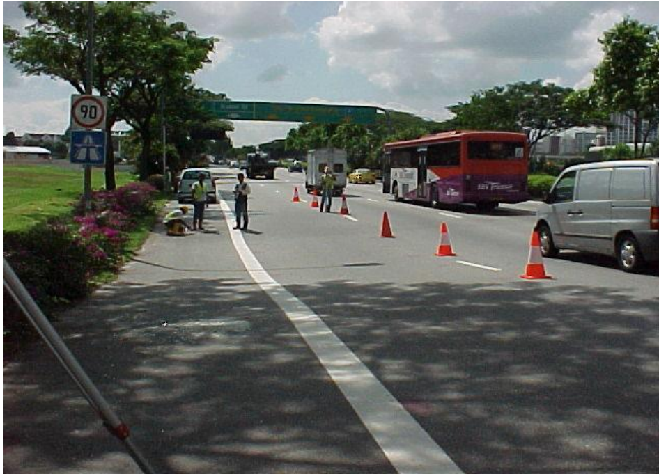
Figure 1.1 Temporary restriction on access to left lane due to ground surface settlement
