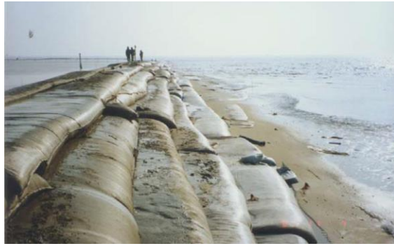
Figure 2.43 A picture showing the formation of a dike using clay slurry filled geotubes (after Yan and Chu, 2010)
