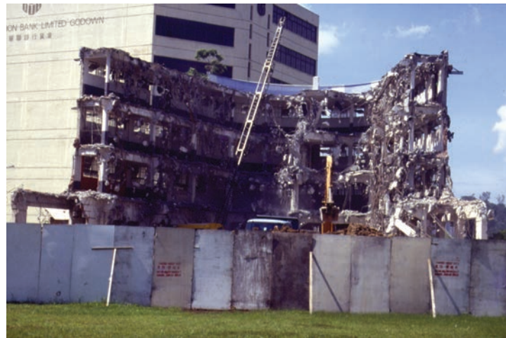
Figure 4.29: The demolition of Hong Bee Warehouse. Kanae Ohgi's HOLE , a mural of blue rectangles in varying tones painted on the rooftop is still visible. Image courtesy of Koh Nguang How
