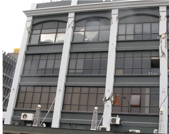
(b) 2011 Christchurch Earthquake, New Zealand
