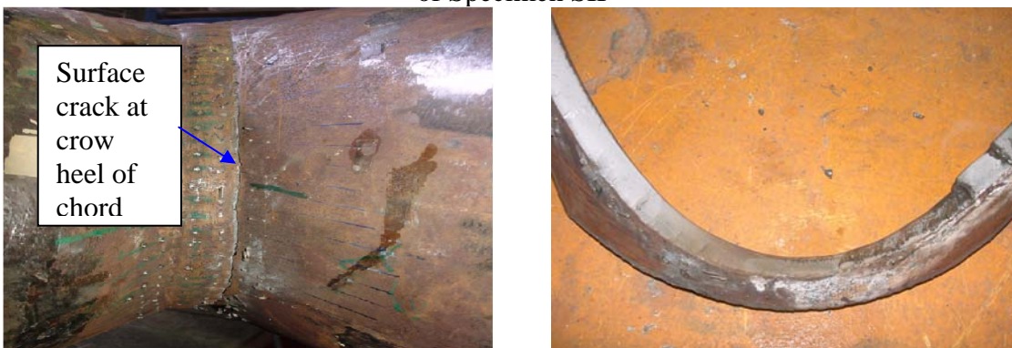
(b) Close-up view and opened surface crack at crown toe of through brace of Specimen SII
