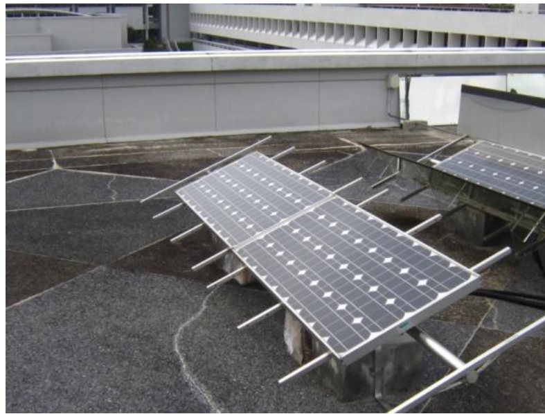
Fig. 3.6 PV modules installed on the building rooftop.
