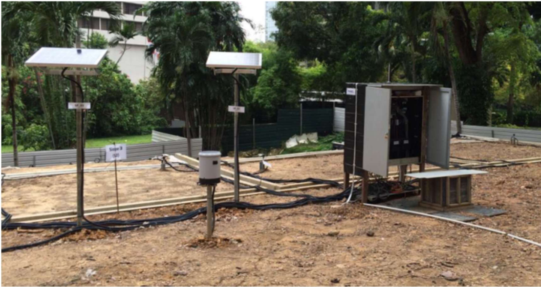
Figure 35: Data acquisition system used at the study site
