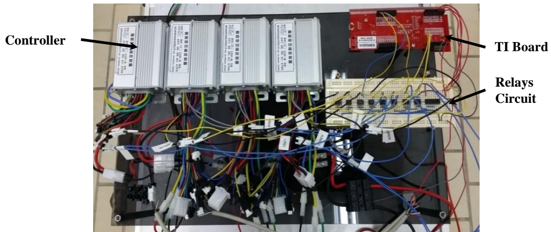
Figure 5.9: Overall view of electronic components
