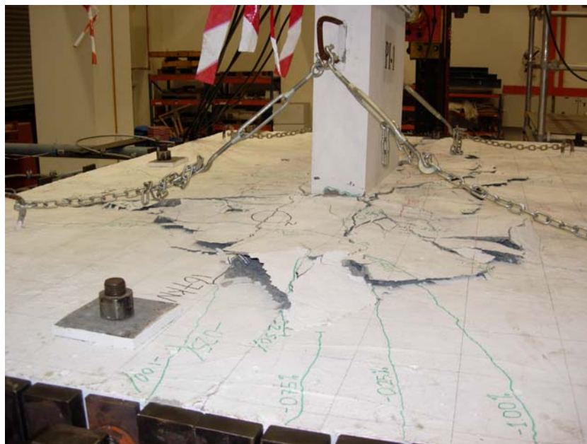
Figure 5.1 Punching shear failure (PI-1)
