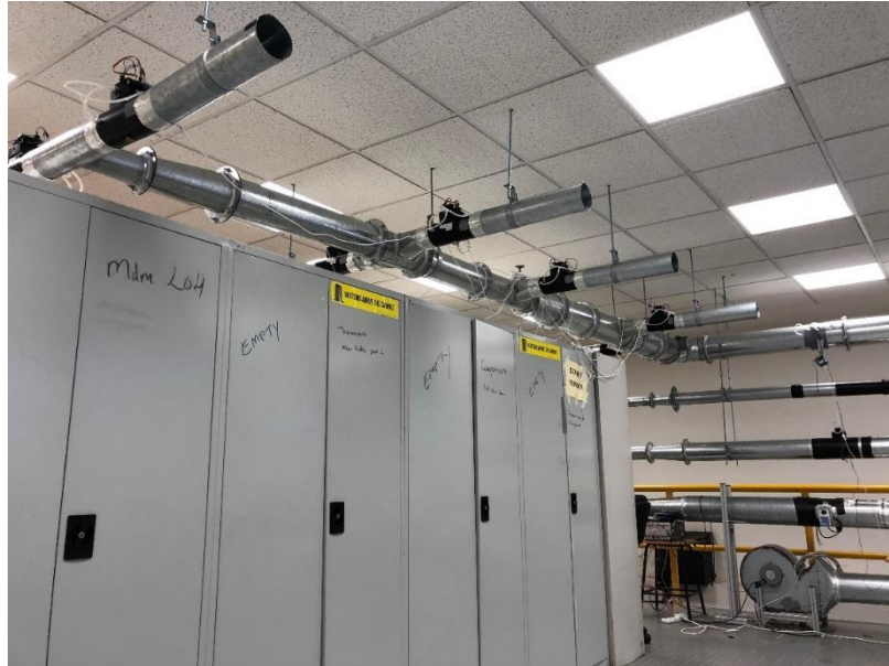
Figure 4.7 Air distribution platform
