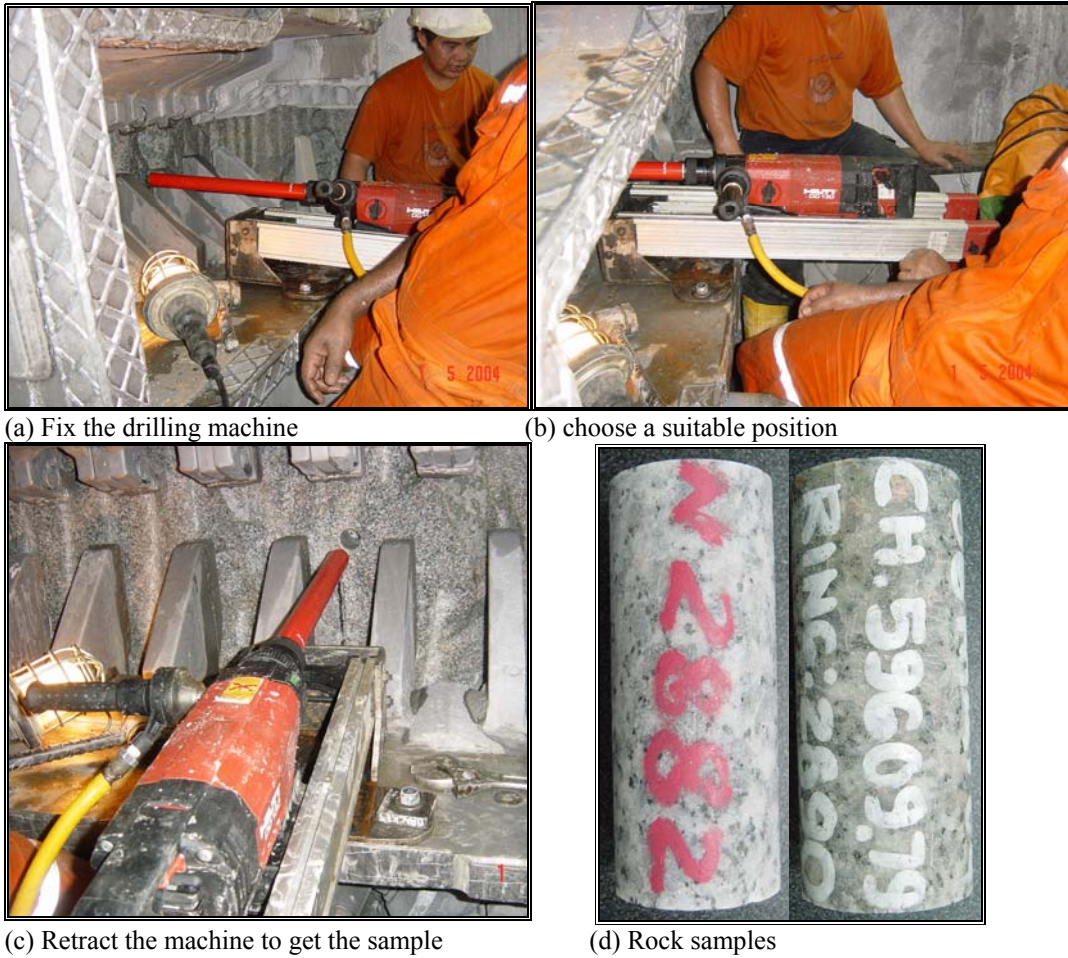
Figure 5.10 Rock sample coring in the tunnel face
