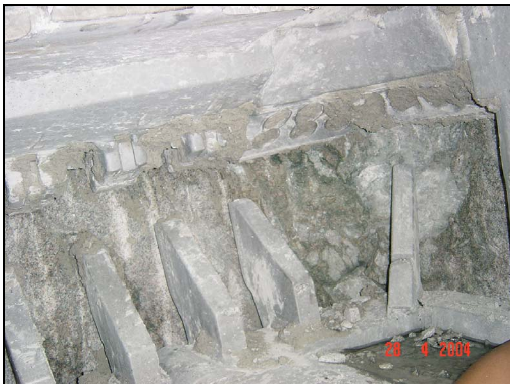
Figure 5.9 Photo taken from the upper right opening of North Ring 2811 in T05
