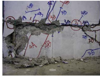
(c) Buckling of reinforcing bars at left bottom column of at DF = \pm 4
