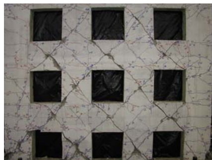
(g) Diagonal cracks at DF = \pm 7
