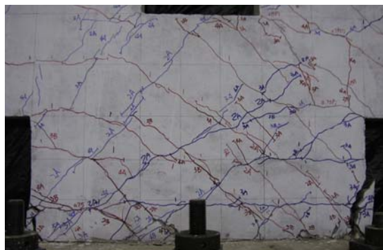
(f) Buckling of reinforcing bars at the bottom panel zone at DF = \pm 5
