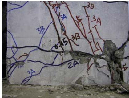
(b) Cracking of bottom right column at DF = \pm 3
