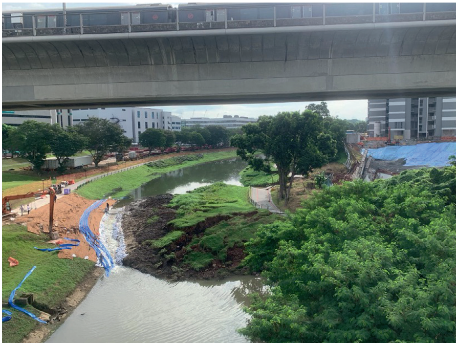
Fig. 1. Landslide on 2 September 2022 at the Clementi construction site, Singapore.
