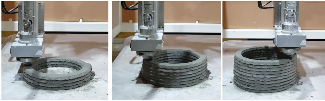
Figure 5.14 3D printing of clay modified geopolymer showing excellent buildability (no visible standoff distance)
