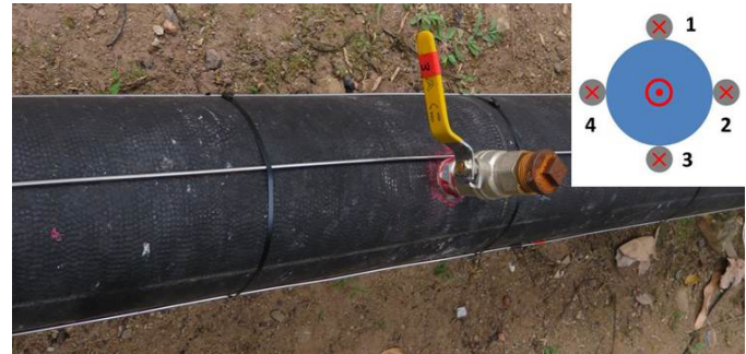
Fig. 7: Installation of DTS sensing cables on the surface of DI pipe. Inset: view of cross section
