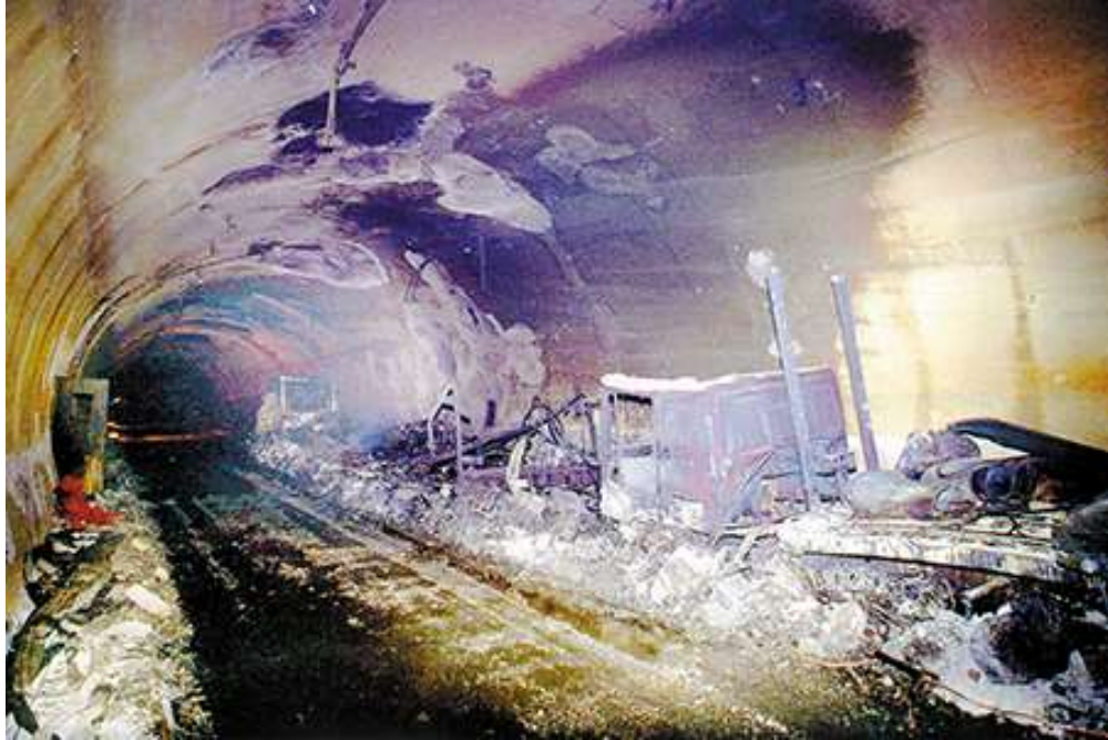
Fig. 1.1 Occurrence of spalling in Mont Blanc tunnel fire (Promat, 2017a)
