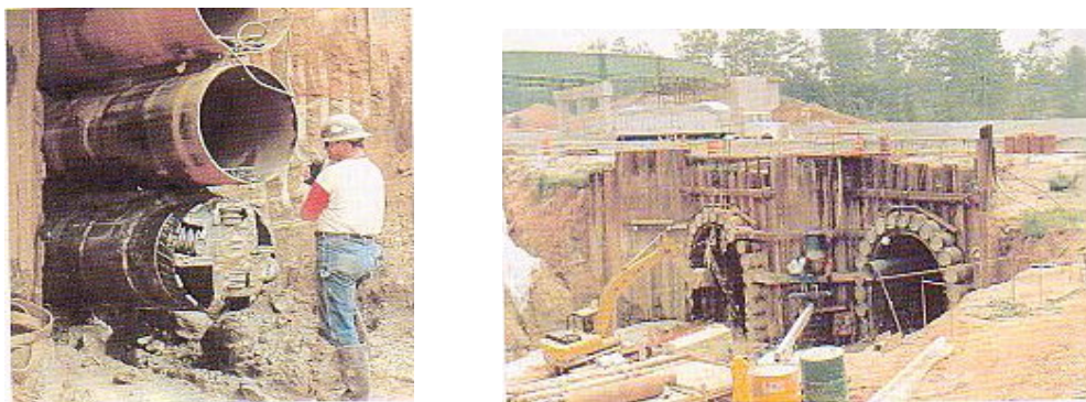
Figure 2-12 and 2-13. Large diameter pipe roofs arranged in an arch shaped umbrella. (McFeat-Smith, 1997)
