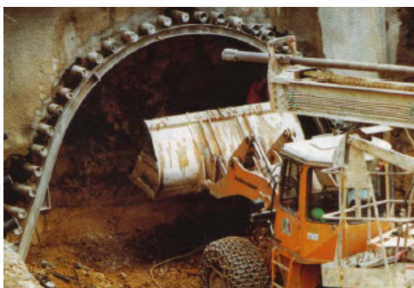
Figure 2-11. Forepoling works in a tunnel in Switzerland (steel ribs are used as additional support).
