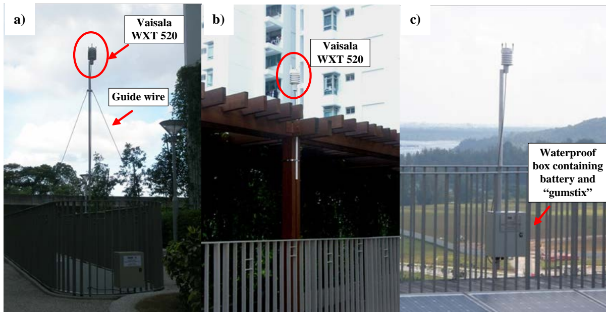
Figure 3.6 a) The Vaisala station installed on the pole; b) the Vaisala station installed on the trellis; and c) the Vaisala station installed on the roof.
