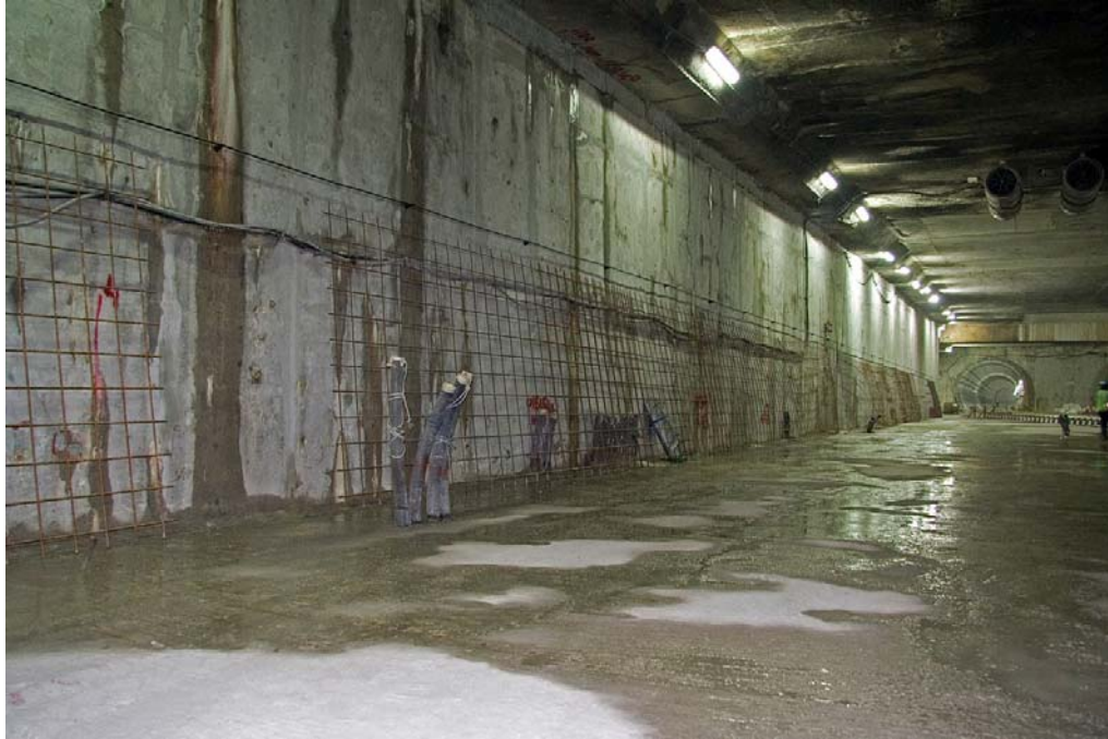
Figure 8.1 Leakage in Cut-and-Cover Tunnel at Dhoby Ghout MRT Station
