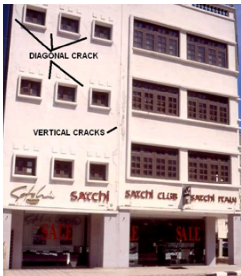
Figure 5.20 Diagonal and Vertical Cracks at Satchi Club
