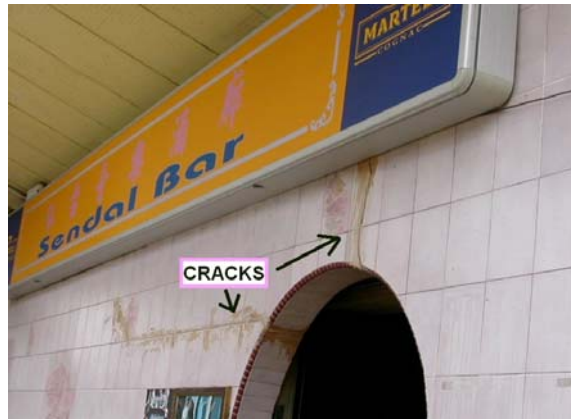
Figure 5.15 Cracks at C706C-a (Sendal Bar)
