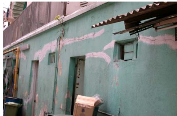
5.16 Typical Cracks Occurred behind Shop Houses C706C
