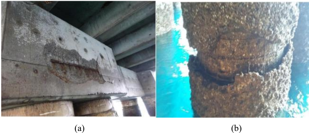
Figure 1.1 Severe corrosion observed in (a) concrete pile cap and (b) concrete jacket after long-term marine exposure (Darmawan et al., 2024).
