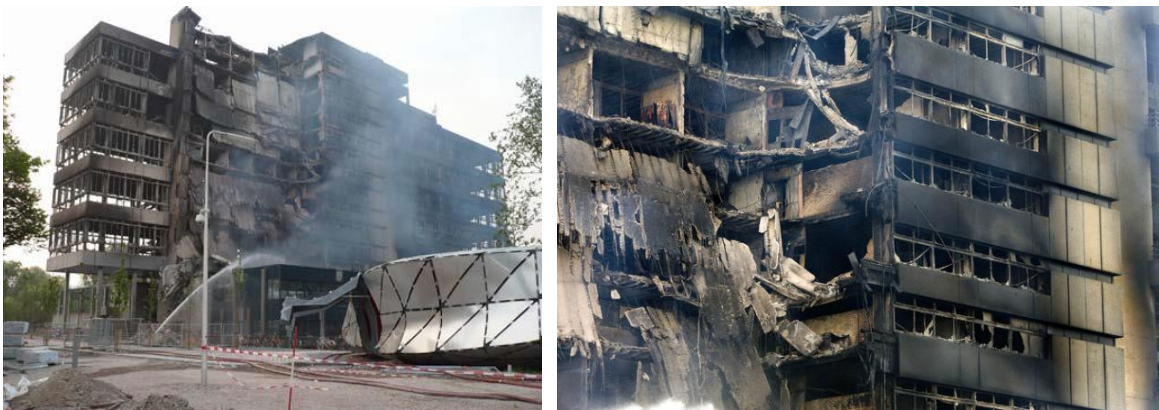
Fig. 1.3. Damage to a multi-story building of the Faculty of Architecture in Delft University of Technology, Netherlands.
