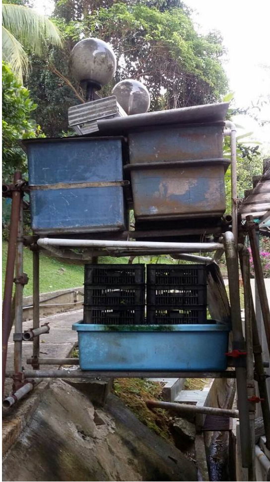
Figure 2.1: Set-up of a handmade filtration system by Jerome Ng for his koi pond. Water passes through the white-PVC pipes through the large plastic tubs, and are allowed to drip down below through the plastic baskets that hold yet more filter material. (Photo credits: Jerome Ng).
