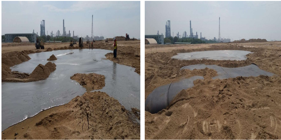
Figure 6.45 Photo showing containment of the slurry seepage from day 1 using sand bund
