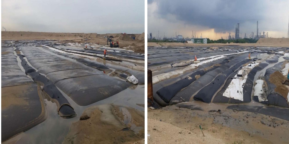
Figure 6.41 Two stage geotube placement at 12m and 5m spacing in stage 1 & 2 respectively
