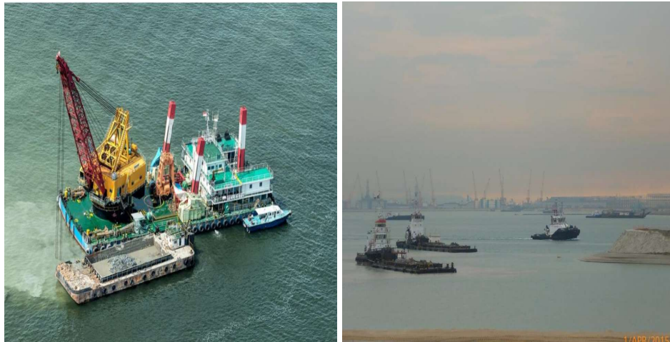
Figure 6.9 Grab dredger loading dredged materials into dump barge (left) and dump barges moving into position over the underwater containment facility for direct dumping (right)
