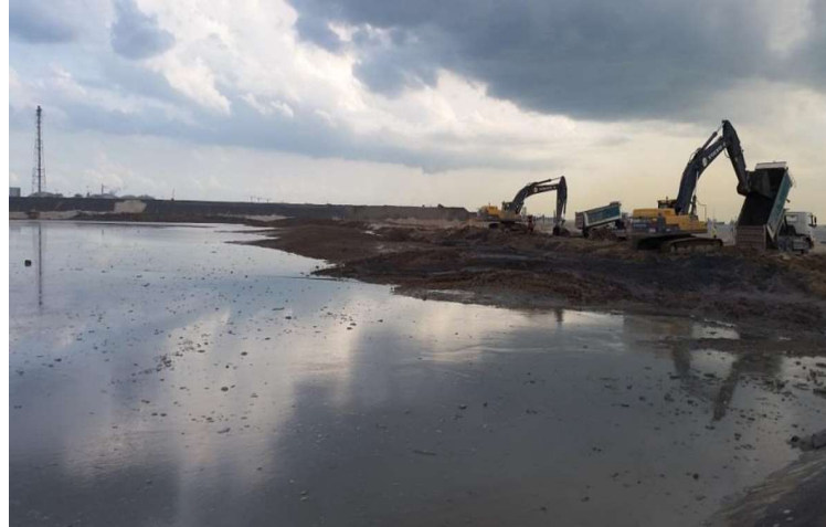
Figure 6.15 Filling and spreading of good earth by trucks and excavators from the sides of the inner containment bund
