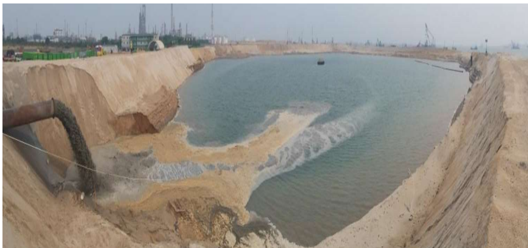
Figure 6.11 Dredged slurry pumped from CSD and poured into the confinement facility as fill
