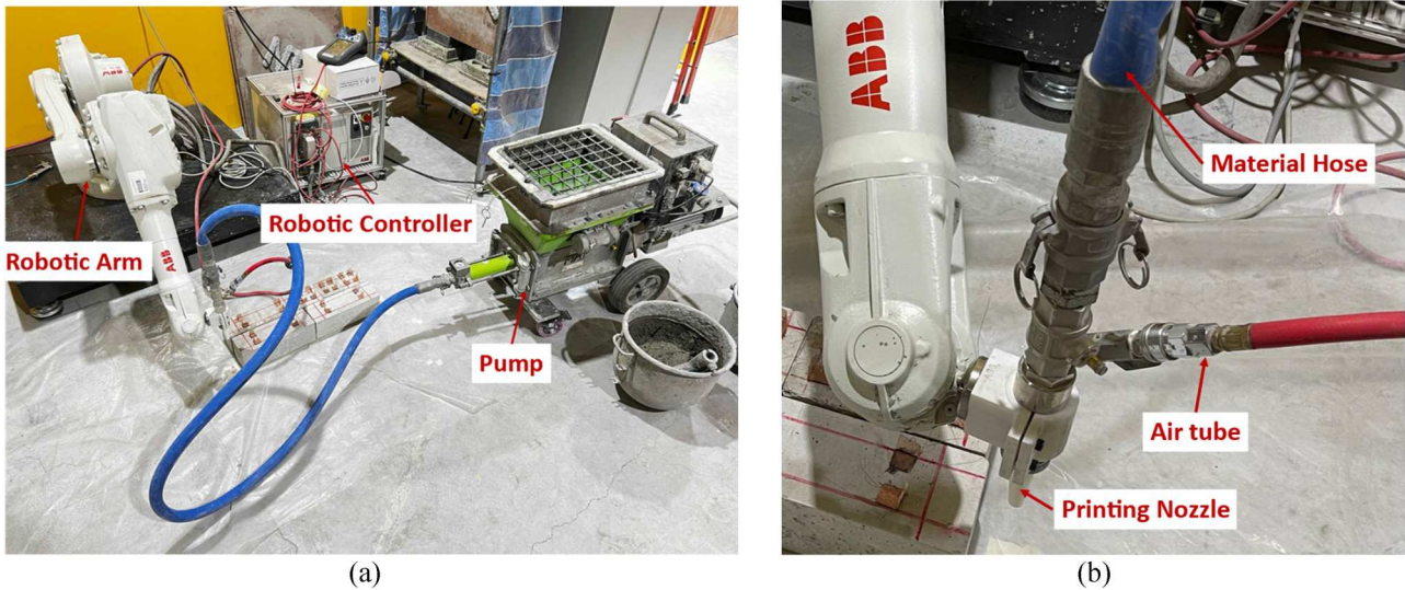
Figure 2. Setup of the robotic spray: (a) spray printing system and (b) details of the spray nozzle.
