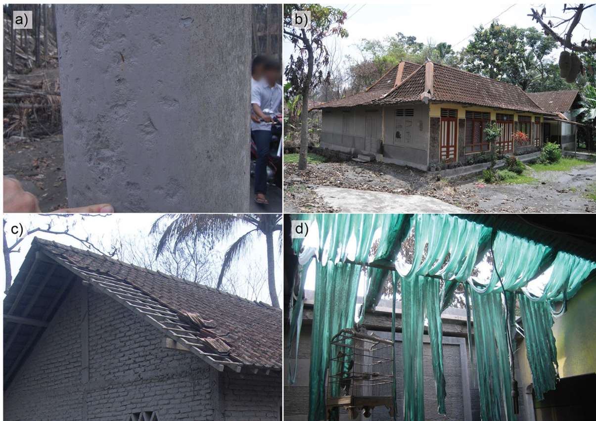
Fig. 7. a) ~7.5 m high concrete utility pole at the base of the concrete levee bordering the Gendol channel showing pockmarks on the upflow side, from small clasts carried within the Leds striking the pole; b) Traditional Javanese building at the edge of Bronggang village showing the very sharp Leds boundary, with ash and dried vegetation from the Leds visible on just the upflow (left of image) wall and surrounds; c) Roof tiles lifted on the overhang of a building facing the direction of Leds overspill suggesting dynamic pressures of ~0.1 to 0.2 kPa; d) Corrugated plastic roofing sheets melted by the Leds and/or the deposits suggesting temperatures of at least 100 °C sustained for ~three minutes. Photos taken by S.F. Jenkins, November 2010.
